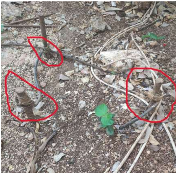
Figure 2. Connection between the electrode and the grounding conductor; it can be seen that only one of the three electrodes has its mechanical connector Own Elaboration
