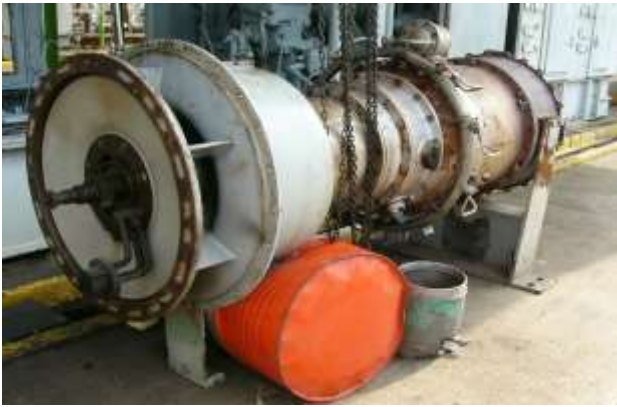
Figure 1 Gas turbine inlet air
