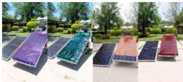
Figure 3 Purple, green, orange and red cellophanes, installed in the MFV Own Elaboration
