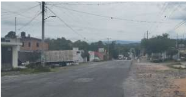
Figure 13 Current road condition from San José Atlán to the expansion section to 4 lanes
