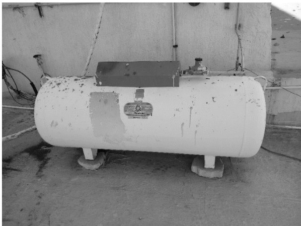
Figure 4 Clinic's stationary LP gas tank for restaurant and laundry use Source: Own elaboration
