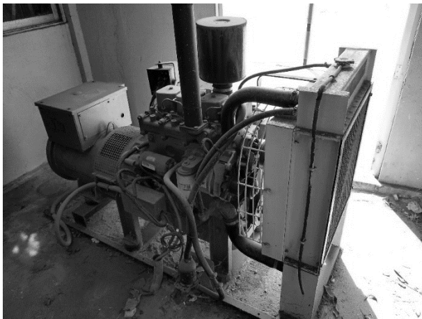
Figure 3 Emergency electric generator of the clinic, operated with diesel Source: Own elaboration
