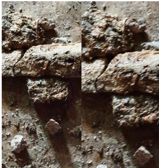
Figure 3.1 Solidified grease extracted from the drainage, causing obstruction and bad odors, this was due to the direct discharge of used vegetable cooking oil from a dwelling house into the sink
