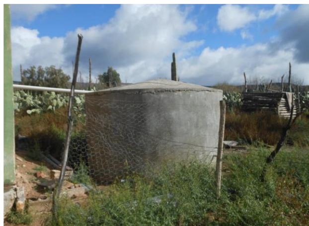
Figure 7 Storage tank type
