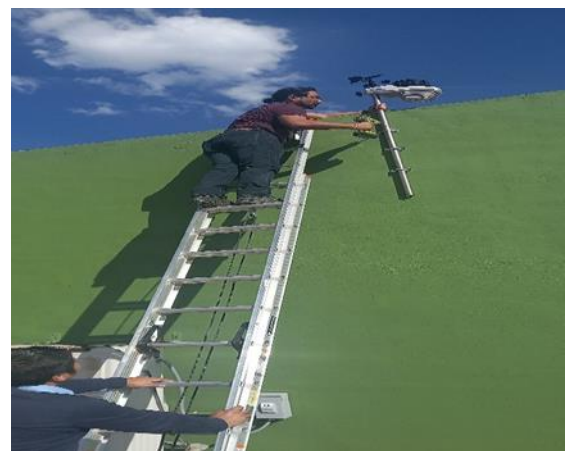
Figure 1 Weather station installation.
