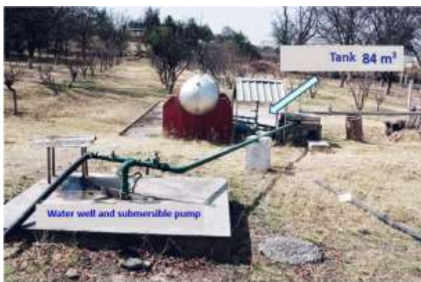
Figure 2 Well, submersible pump and reservoir Source: Own Elaboration
