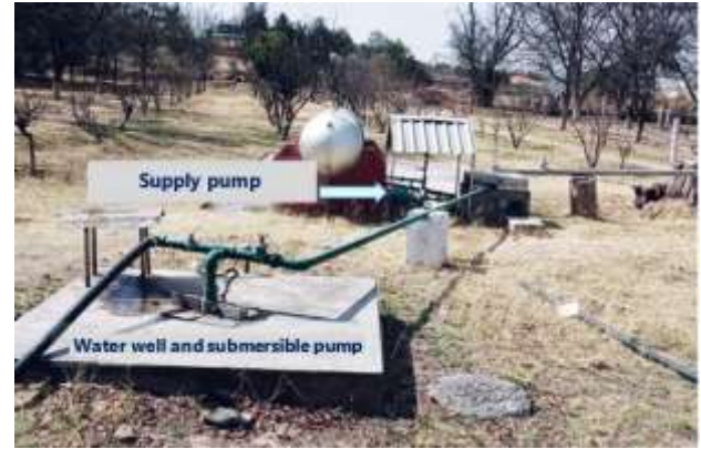
Figure 3 Well, submersible pump and supply pump Source: Own Elaboration
