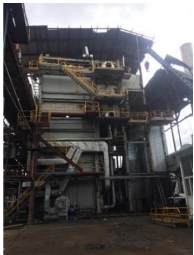
Figure 1 La Joya sugar mill baghouse boiler Source: Own elaboration.
